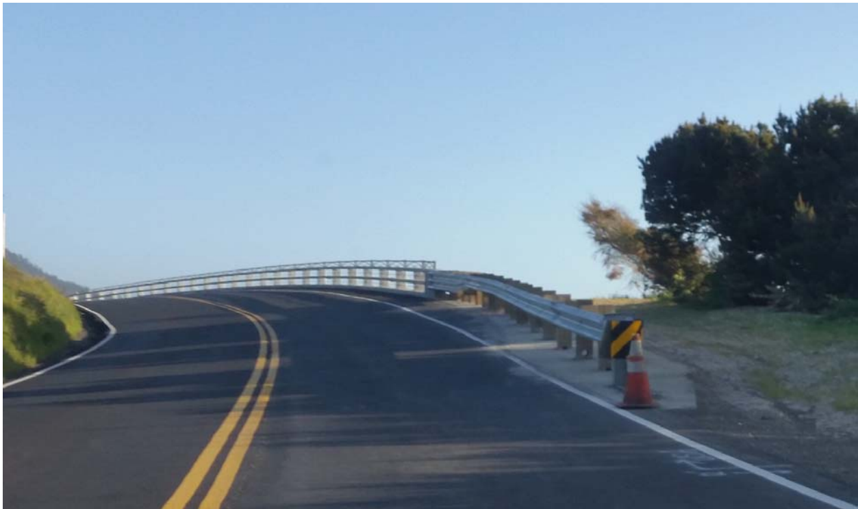
Close up showing proximity of north end of guard rail to the fog line.
